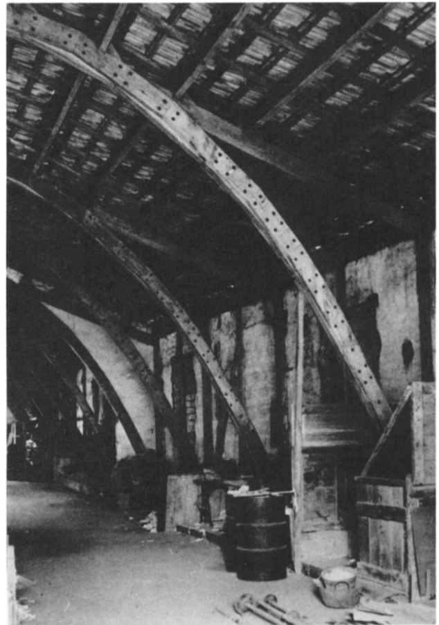
Fig. 3. Antoni Gaudí, Machine Hall, Mataró. Interior (photo: courtesy Gaudí Archive, Columbia University).
